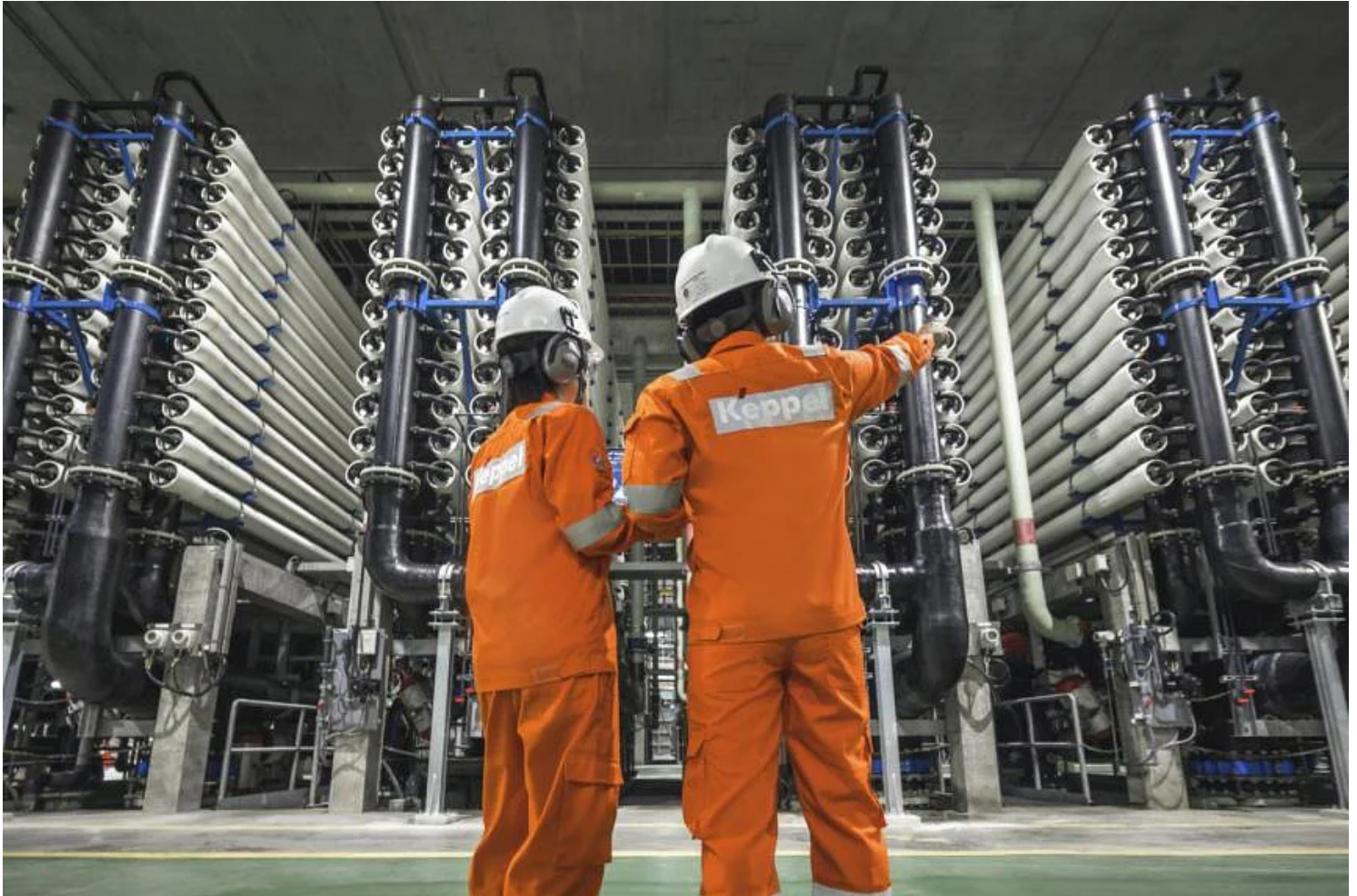
The Keppel Marina East Desalination Plant was one of three PUB projects that won gold awards. PHOTO: KEPPEL CORPORATION
